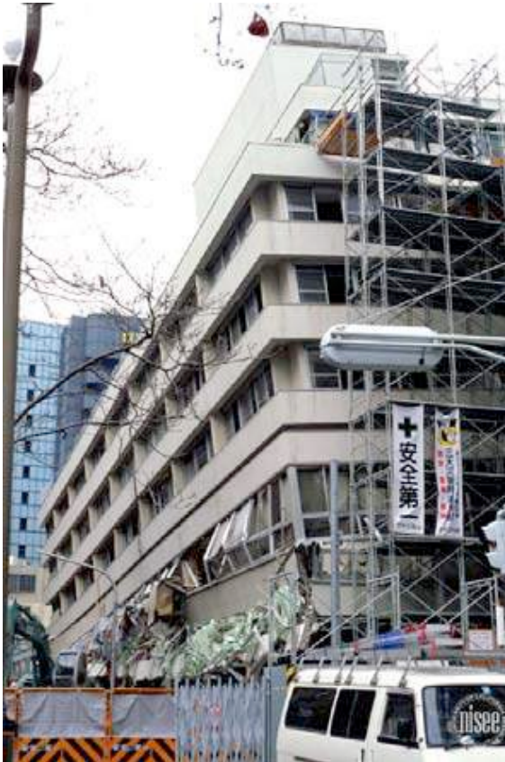
Figure 1. In 1995 Kobe Earthquake, the first and third floors were collapsed totally because of irregularities in planning between adjacent floors of building. In Kobe earthquake, the total collapse of the ground floor depends on the soft layer arrangement in architectural planning. (Clark, W. Peter, Kobe Collection, Nisee) (Nisee http://nisee.berkeley.edu/images/servlet/EqjisDetail?slide=K0068 ).
