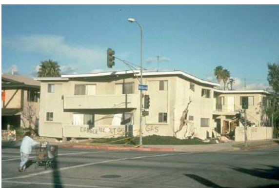
Figure 2. The collapse of the apartment on the ground floor depending on the effect of soft floor arrangement. (California earthquake in, 1994, Northridge).
